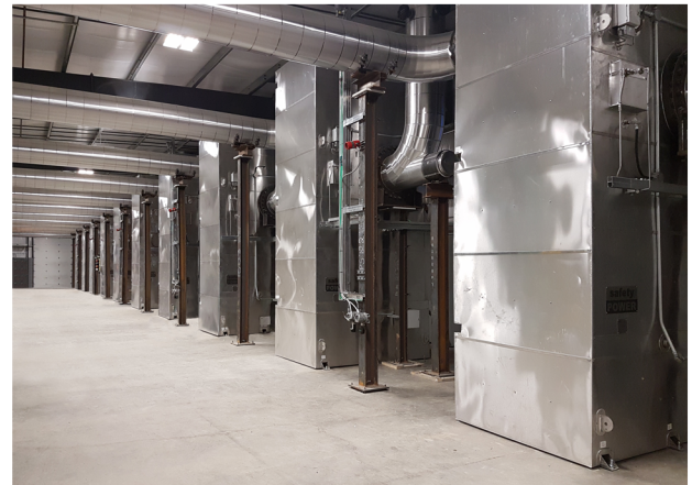
20MW Peaker plant equipped with vertical ecoCUBE® SCR systems
