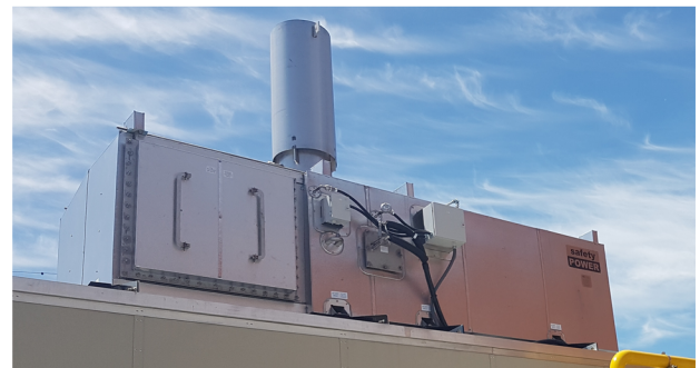
One of twenty enclosure mounted ecoCUBE® installations for Peak Shaving with major national retailer
